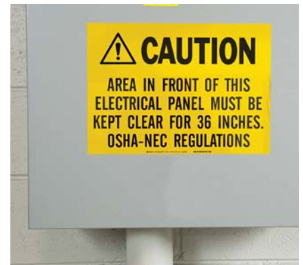
Hazard warning signs
