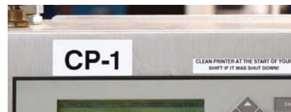
Control Panel & Electrical Panel Labels
